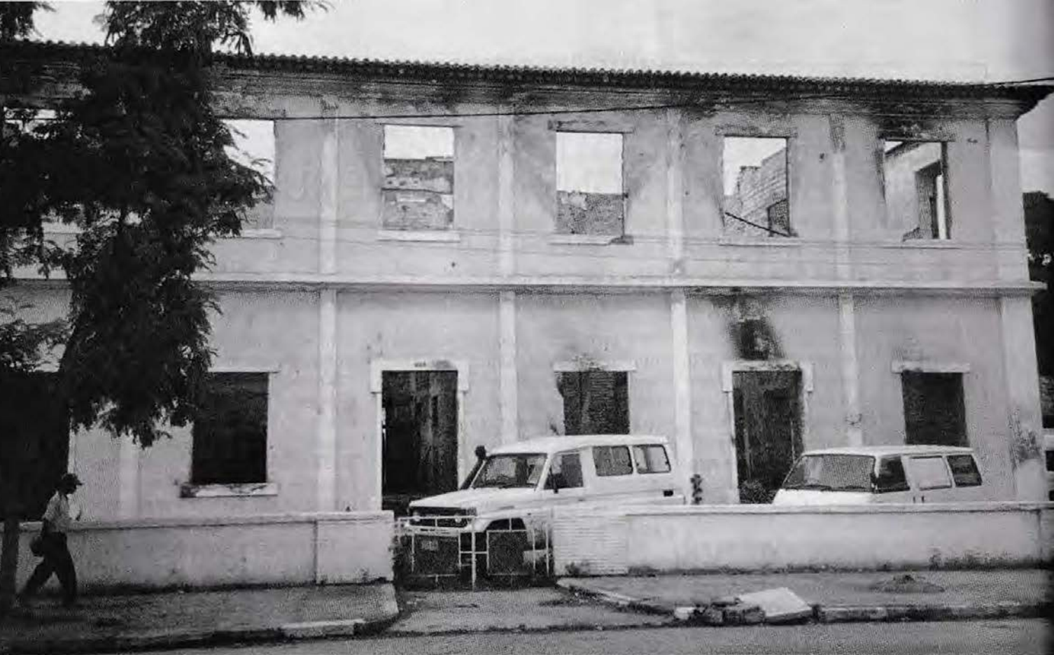
All that remains of the Catholic Church Offices, Dili after the militia set fire to it.
